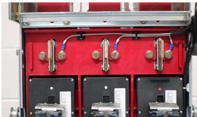
Line-side voltage connections on DS Breaker (Fingers Removed)
